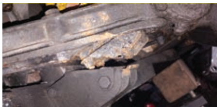
5. A bump stop was missing and had to be replaced.
